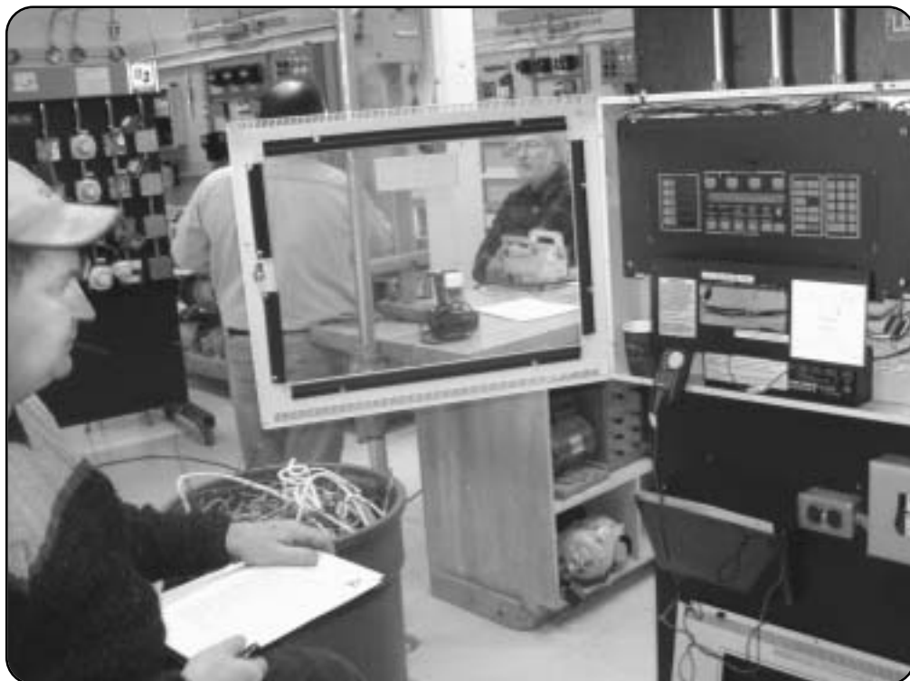
Level 4 Fire Alarm Upgrade
